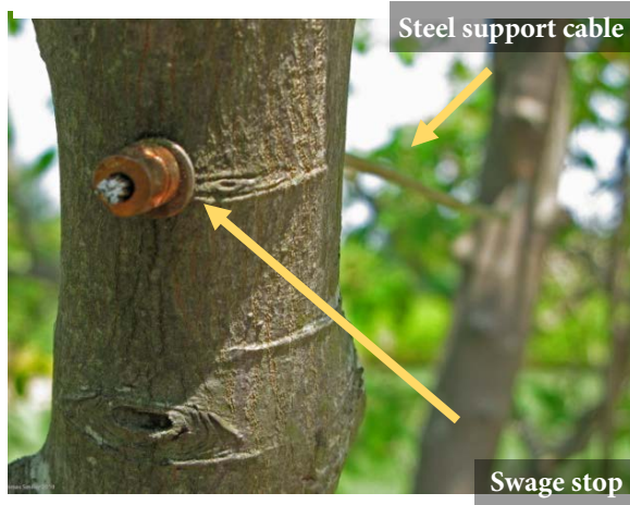
Figure 3: A swage stop-fastened cable system is used in branches less than 3 inches (75mm) in diameter
