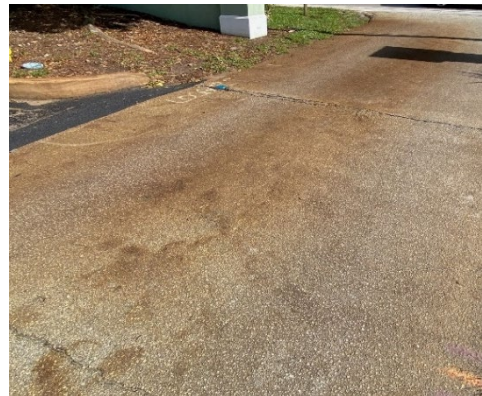
Figure 1: Surface staining below the canopy of an infested black olive tree
