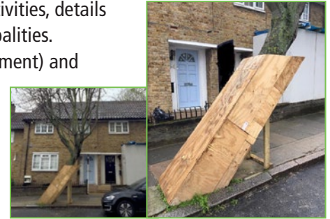
This plywood tree protection box with support was created for a street tree with a 45 degree directional lean.
